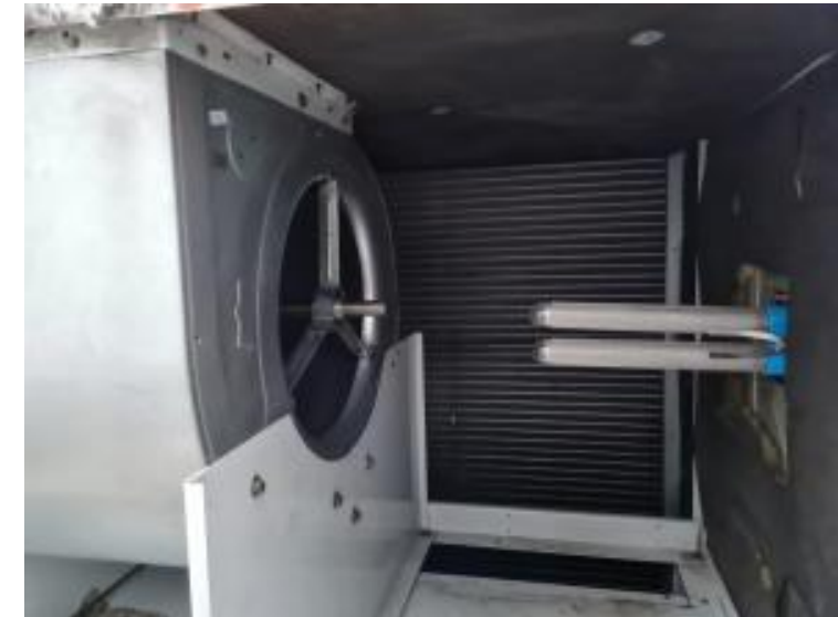
Centralized air condition plasmacluster installed location
