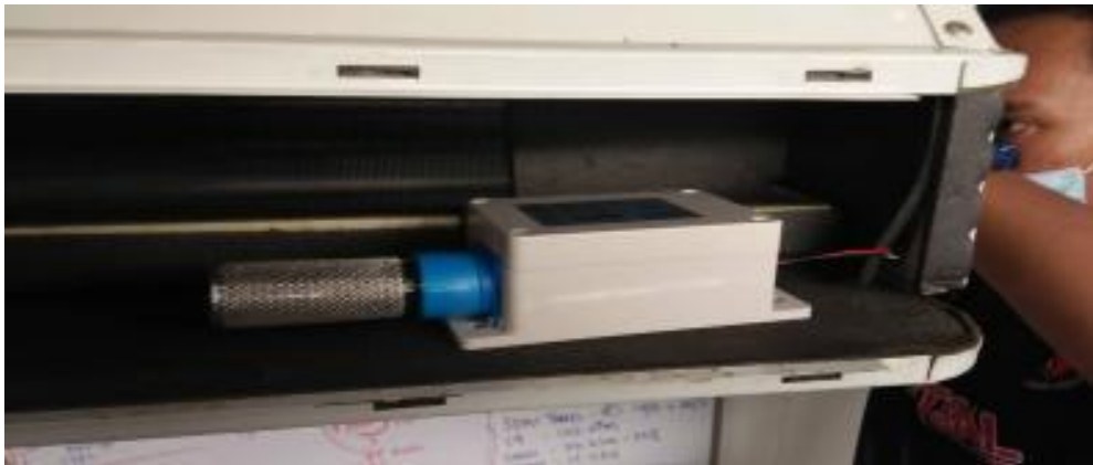
Split unit air conditioner plasmacluster installed location
