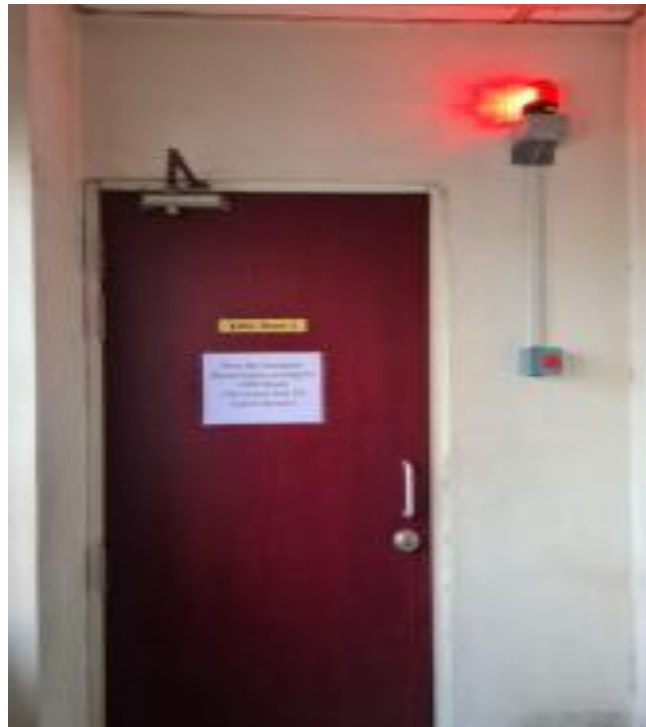
Warning light outside room indicating UVC Light is ON inside AHU Room
