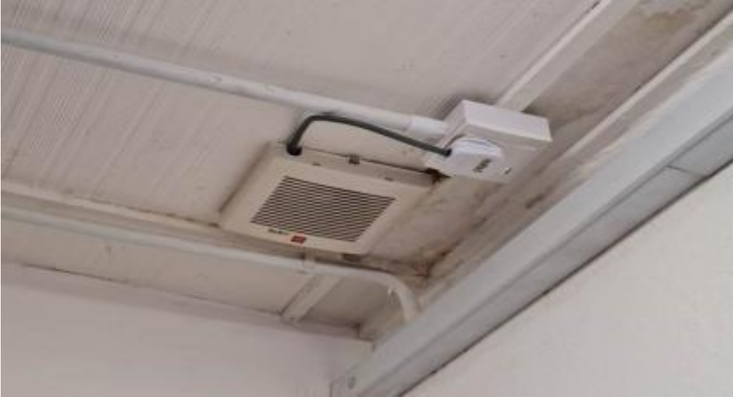
Ceiling mounted ventilation fan
