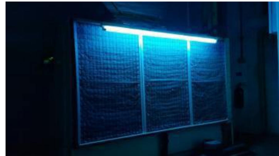
UVC at AHU Inlet
