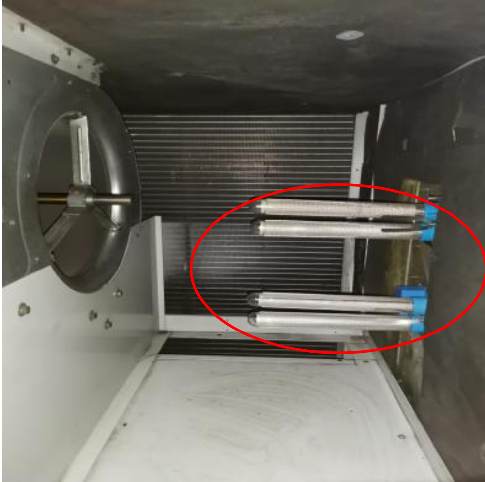
Centralized air condition plasmacluster ionizer installed location
