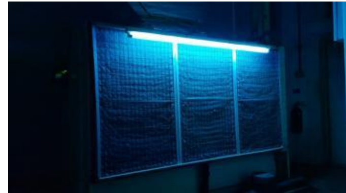
UVC at AHU Inlet
