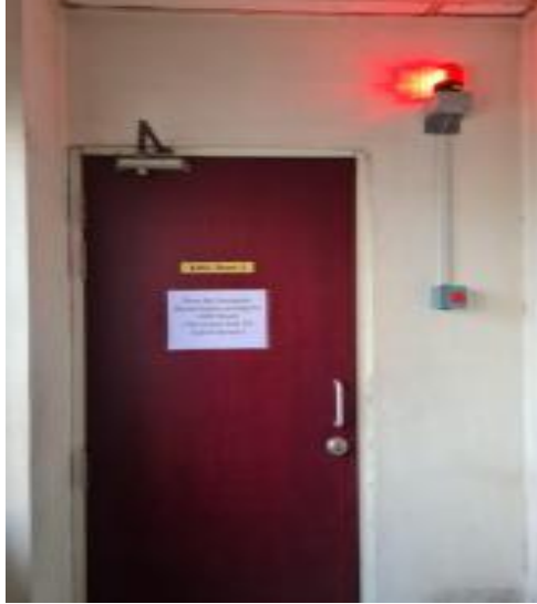
Warning light outside room indicating UVC Light is ON inside AHU Room
